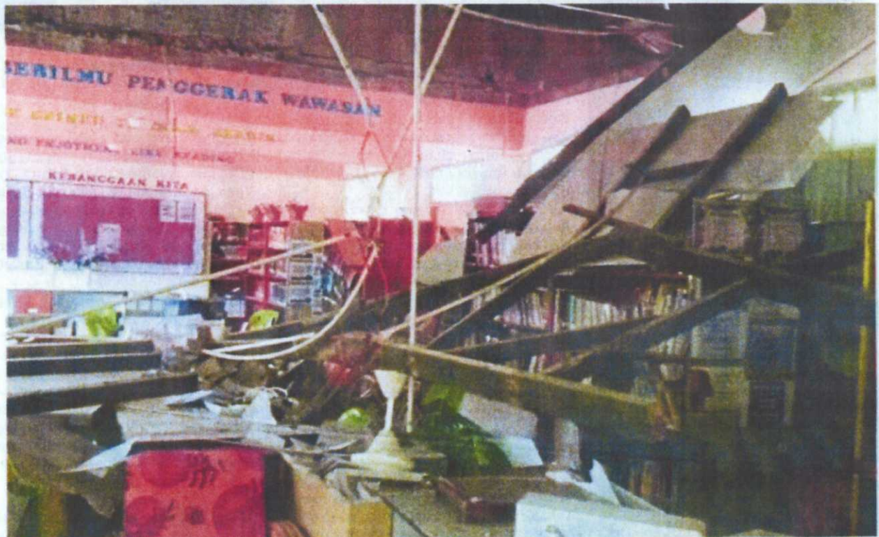
SMK Agama Mohamad Ali's library was damaged in the aftershock yesterday.
